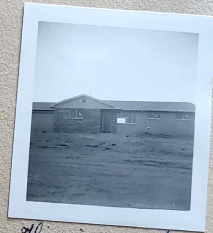
This is a picture of the new parsonage. It is not completed yet but all is going well.
